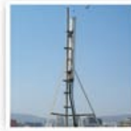
Vodafone Microwave Installation in Mumbai
