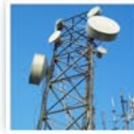
TTML Microwave Installation in Mumbai
