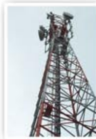
Microwave Installations in Maharashtra & Goa
