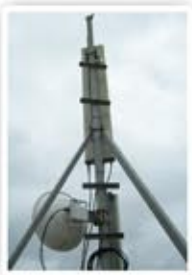
BTS and Microwave Installation in Mumbai
